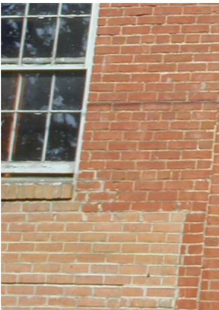
The patchwork on this brick building is evident by the difference in the color of the brick as well as the color, composition, and texture of the mortar.
