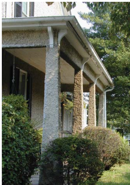
The parging of elements not historically covered in such a material is not appropriate.
