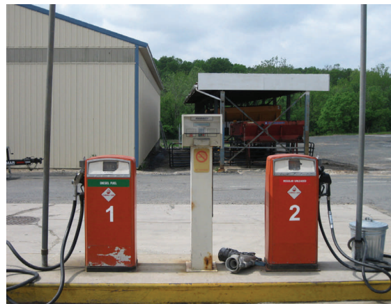
Town Motor Fuel Pumps
