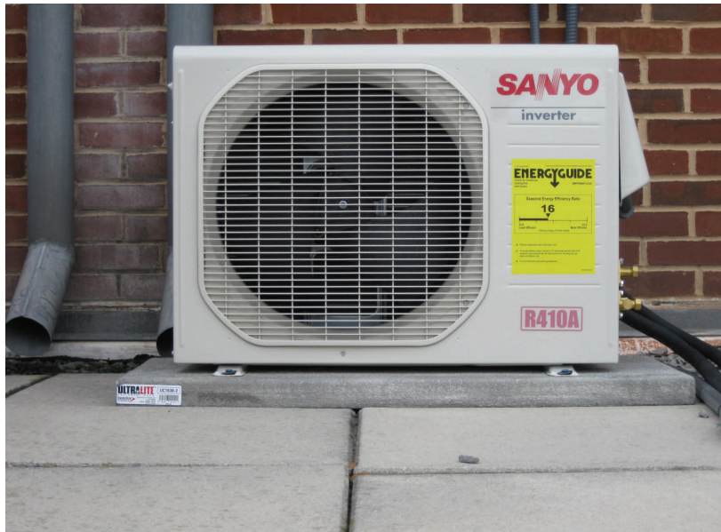
Energy Efficient Inverter added to Town Hall to cool data closet when the building is in setback mode
