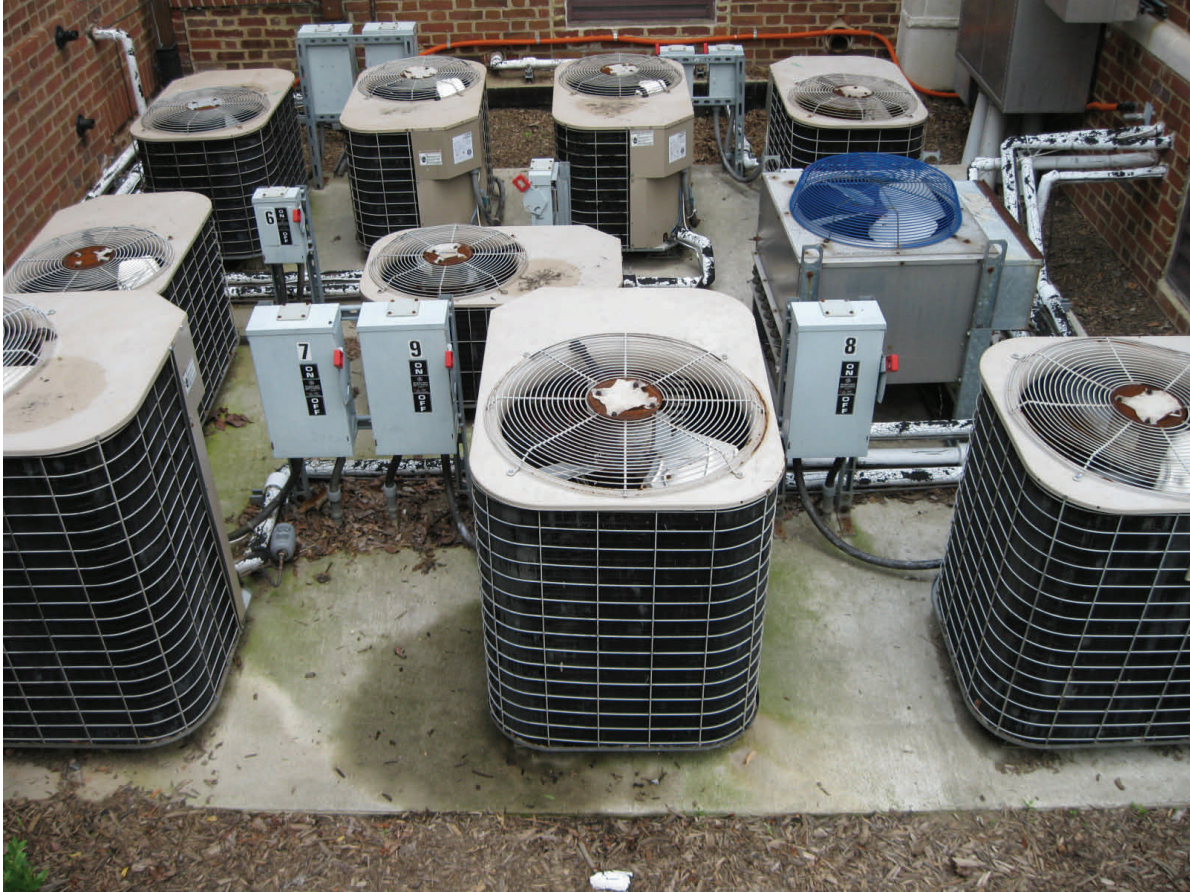
HVAC units at Balch Library
