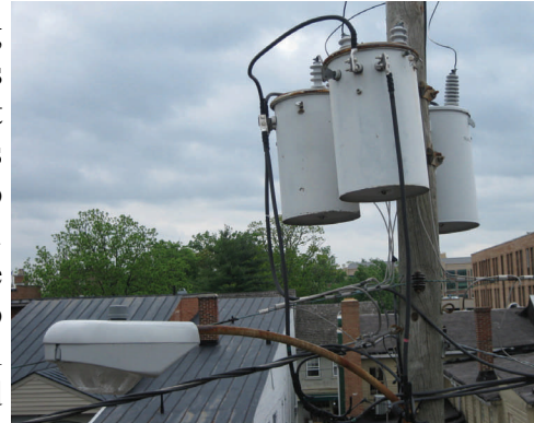
Electric Transformers and Street Lamp
