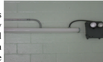
T-5 Fluorescent Lighting at WPCF
