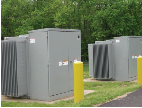
Electrical Transformers at Water Pollution Control Facility
