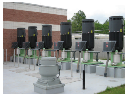
Variable speed pumps at WPCF
