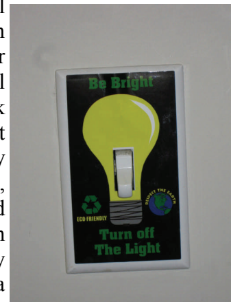
Light Switch at Town Hall
