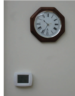
Programmable Thermostats at Balch Library allow setbacks for times when the building is unoccupied
