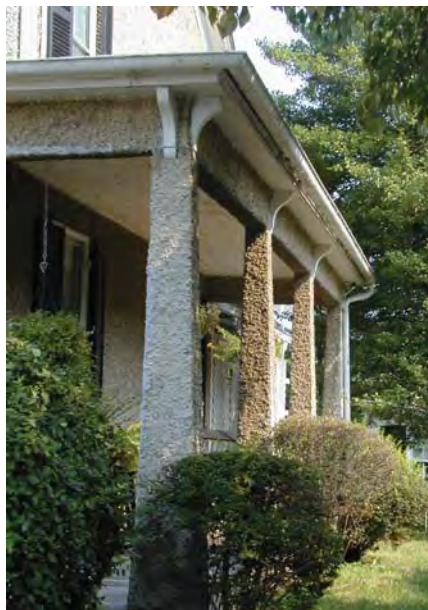
The parging of elements not historically covered in such a material is not appropriate.
