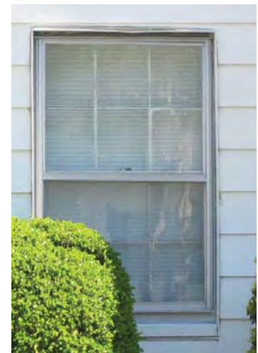
INAPPROPRIATE: Covering over of a window frame, as shown here.
