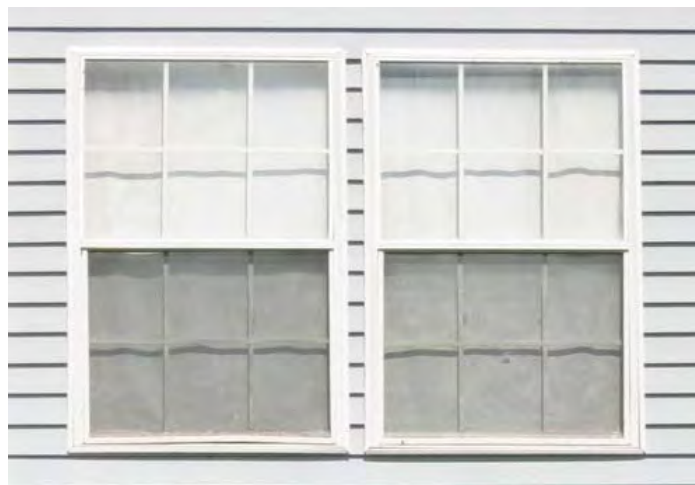
Interior fake muntins do not provide the visual depth and shadow lines found on three-part simulated divided light or traditionally constructed windows.
