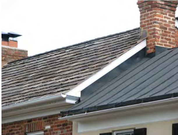
Standing seam metal roofs are prevalent in much of the district, and, in some cases, replaced earlier wood shingle roofs.
