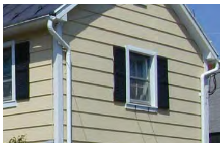
The shutters shown above are the correct size for the opening but are not mounted on hinges and, therefore, do not appear to be operable.
