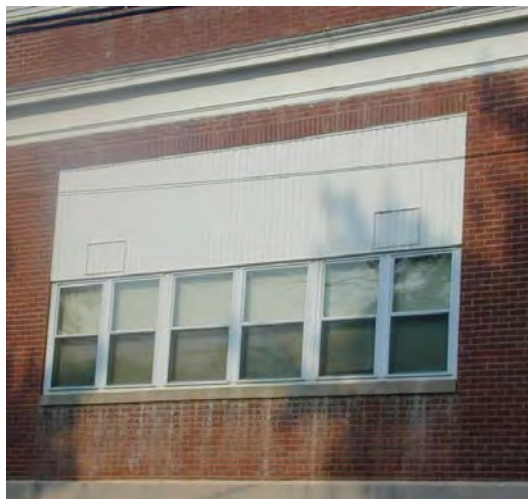
INAPPROPRIATE: Replacement windows should not change the size or glazing pattern of the original windows, as shown above.
