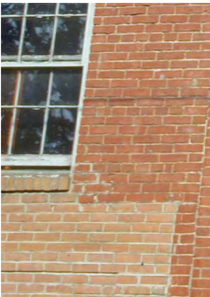
The patchwork on this brick building is evident by the difference in the color of the brick as well as the color, composition, and texture of the mortar.
