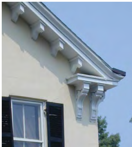
A bracketed cornice return is an important element on this historic building.
