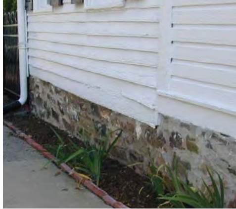
A stone foundation on a historic house clad in wood siding shows historic detailing.
