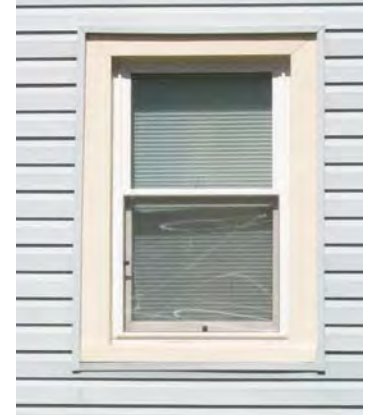
INAPPROPRIATE: Replacement windows should fit the opening; panning (flat inserts around a window) may not be used as a filler.
