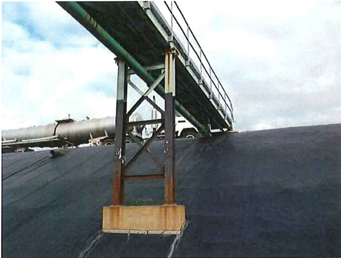
19) Catwalk supports have general surface rusting.
