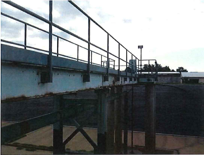
16) The catwalk structural steel and piping coating is in poor condition.
