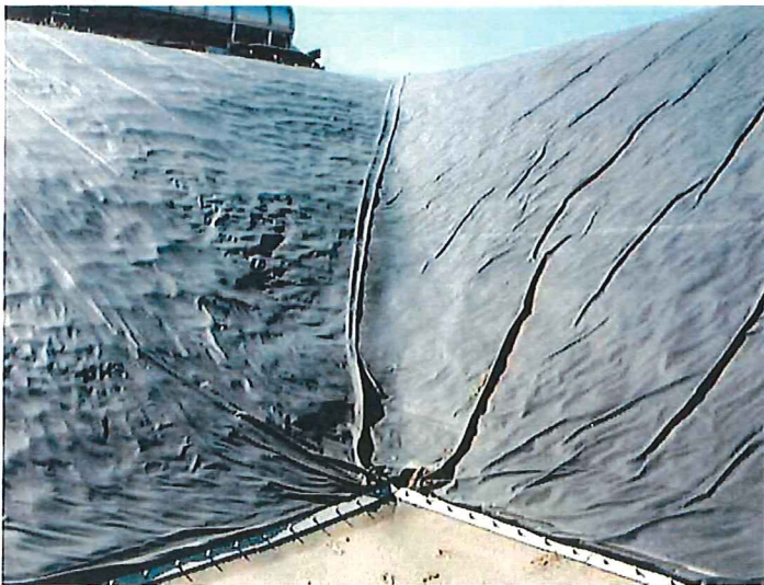
9) Liner is loose and sagging in many areas.
