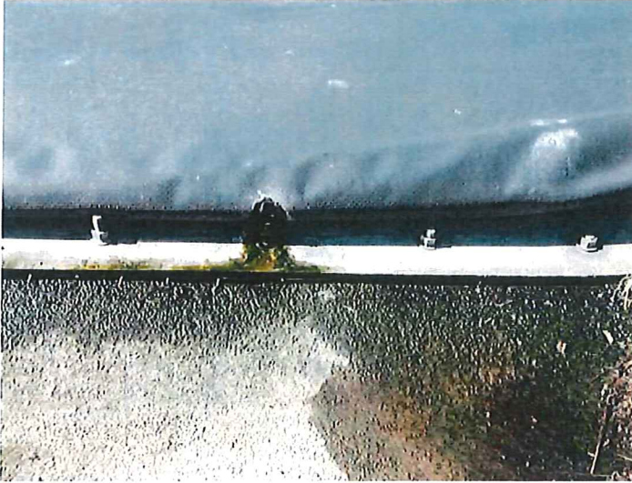
7) Liner is tearing at bolted strips.
