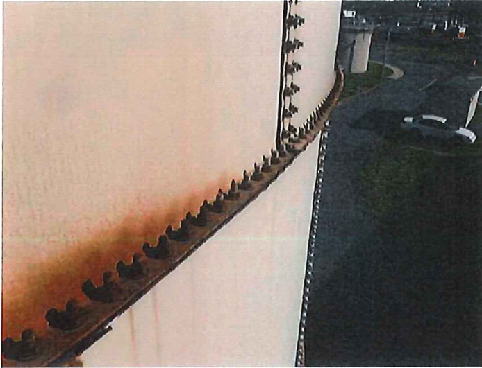
10) Rusting on lip of bolted side-wall stiffener.
