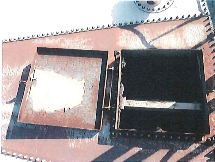
13) Roof cover with coating failures and surface rusting.
