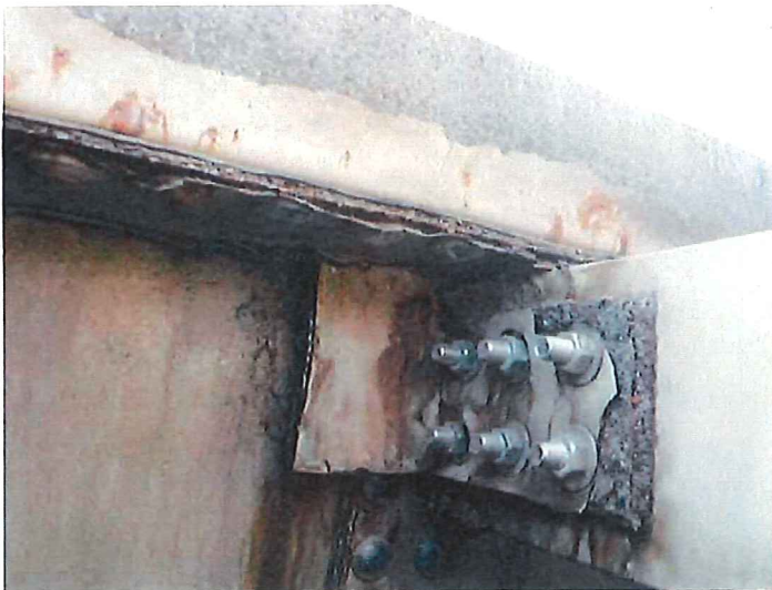
21) Roof stiffeners bolted to sidewall connection plates with coating loss and corrosion forming.
