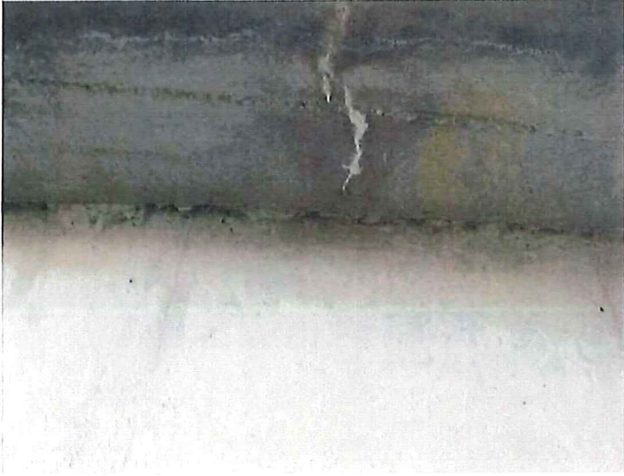
4) Cracking on underside of foundation.
