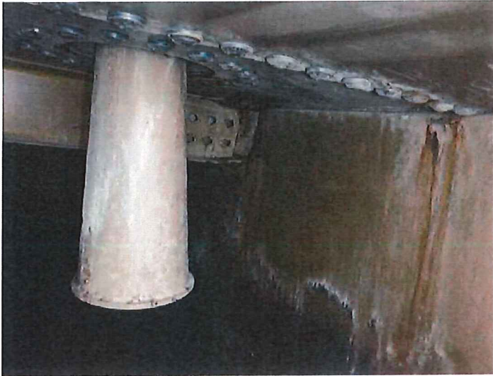
19) Spot coating failures at top of the interior sidewall.
