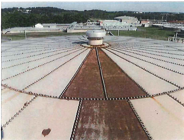
12) Roof panels with surface rusting.
