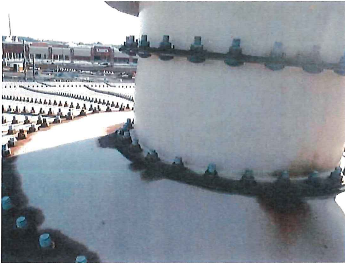
16) Roof vent with rusting bolted connections.
