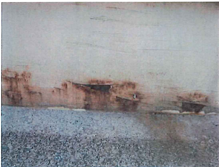
9) Sidewall coating failures above foundation.
