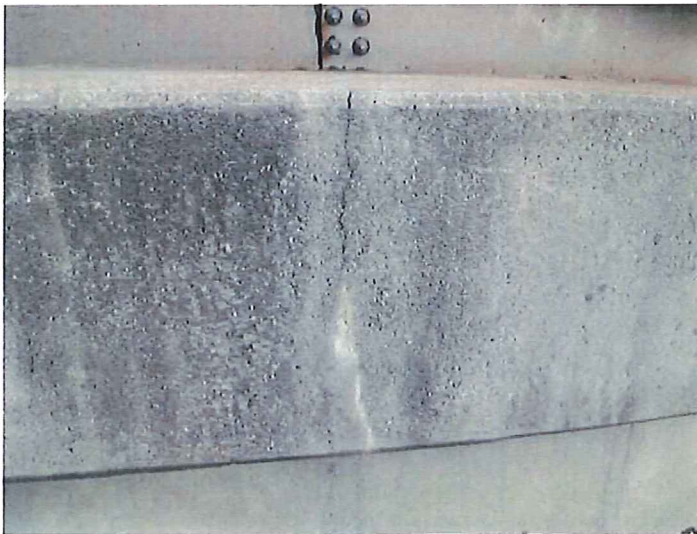
3) Vertical cracking is tight.
