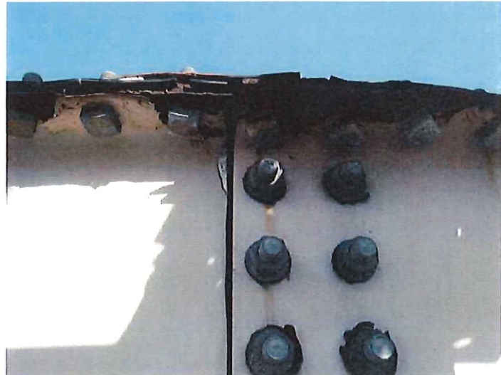
11) Top of sidewall at lip with coating failures and rusting.
