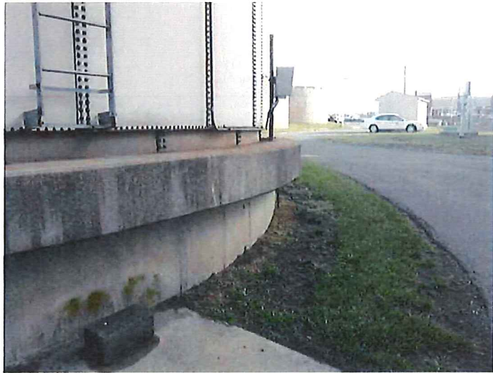
2) Foundation is in good condition with a few cracks.
