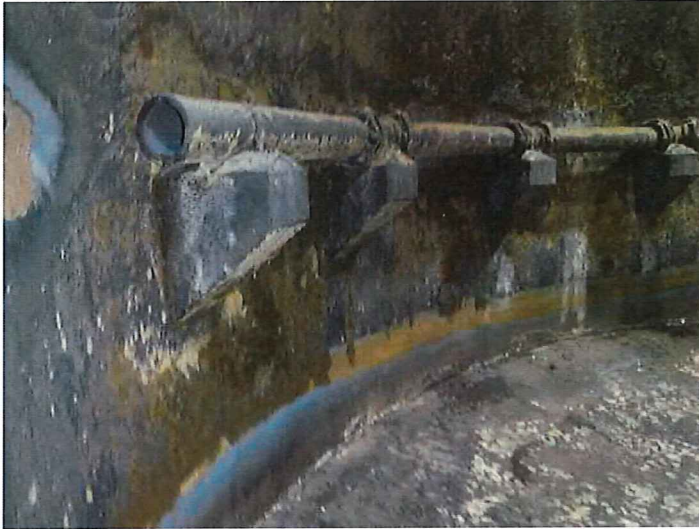
16) Piping mounted on sidewall.
