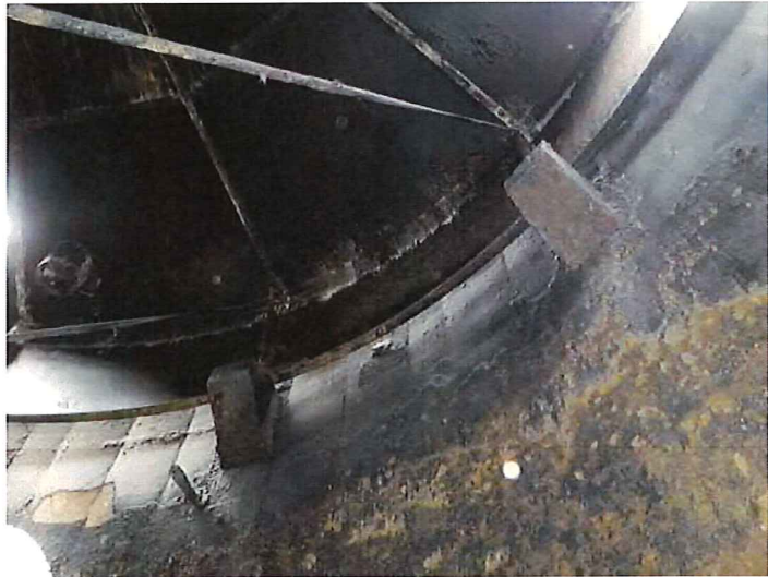
20) Sidewall coating with delamination.
