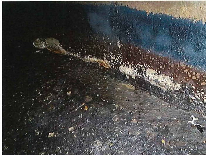
26) Minor concrete spalling at bottom of sidewall.
