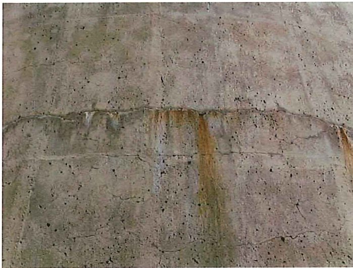
1) Horizontal cracking on the sidewall.
