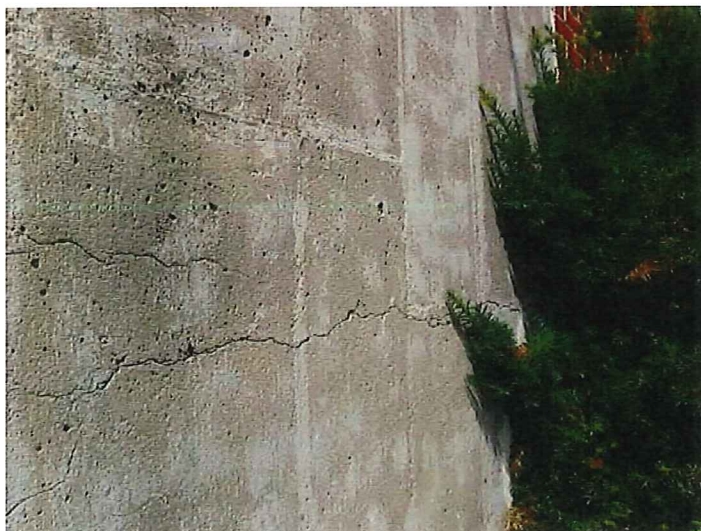
6) Cracking is tight.
