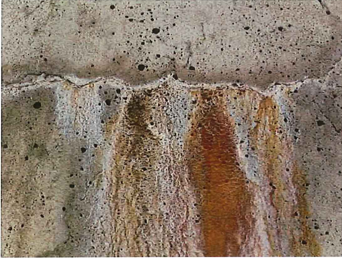
4) Efflorescence and rust staining at cracking.
