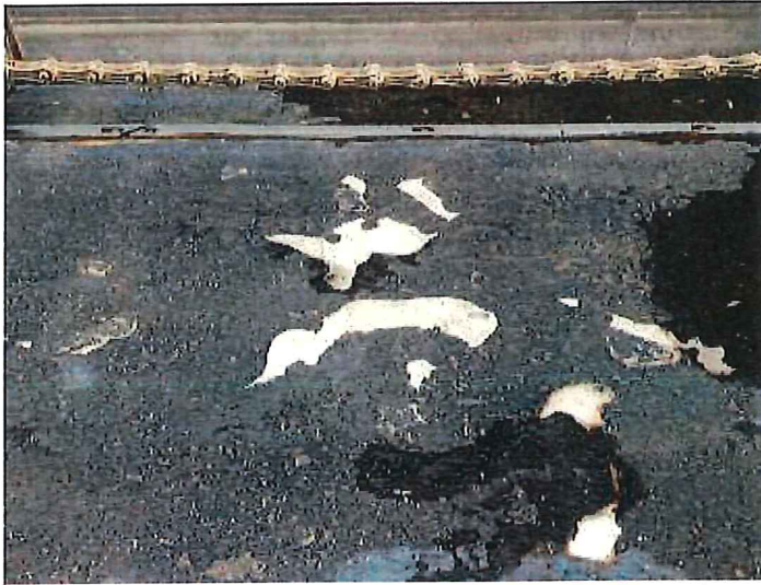
10) Coating failures on the floor.
