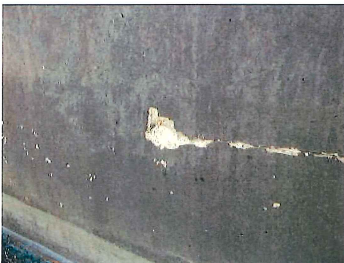
15) Coating delamination on interior sidewalls.
