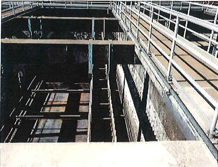
4) Fiberglass launders with weirs.
