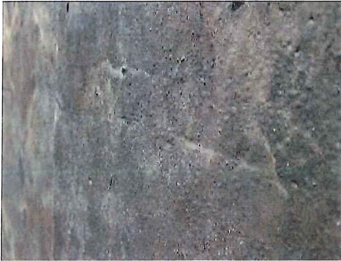
13) Coating blistering on interior sidewalls.
