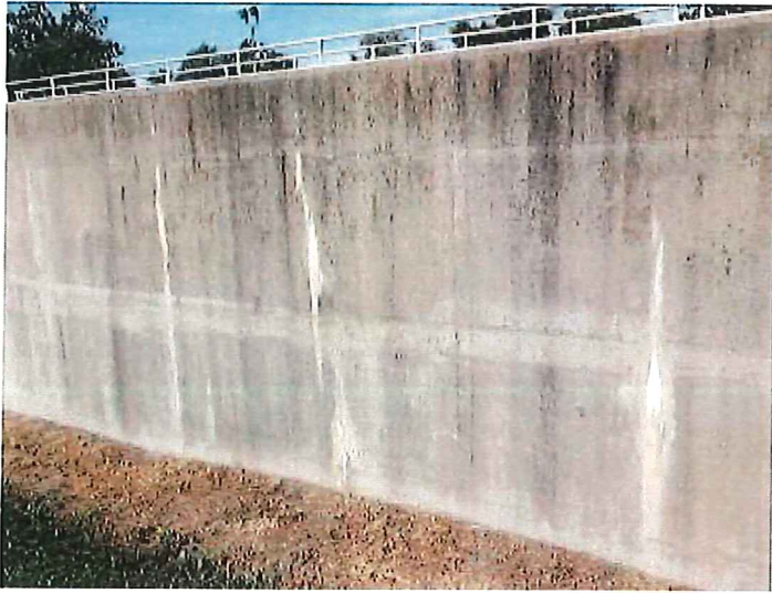
19) Exterior concrete with cracking and efflorescence.
