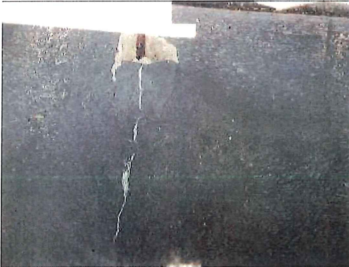
7) Cracking and spalling at top of interior sidewall.
