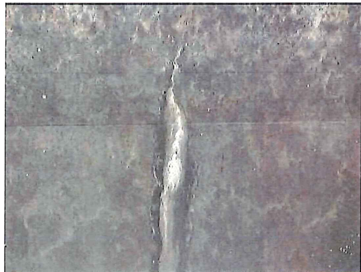
8) Cracking on interior sidewall.
