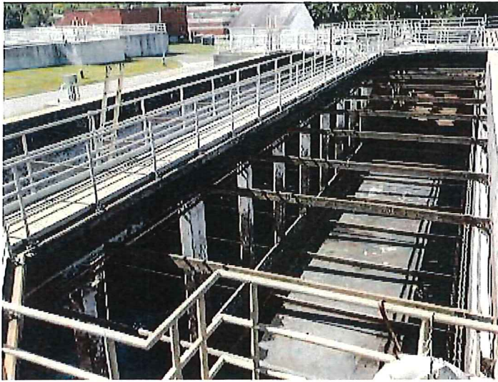
1) Secondary clarifier with catwalk and support steel.
