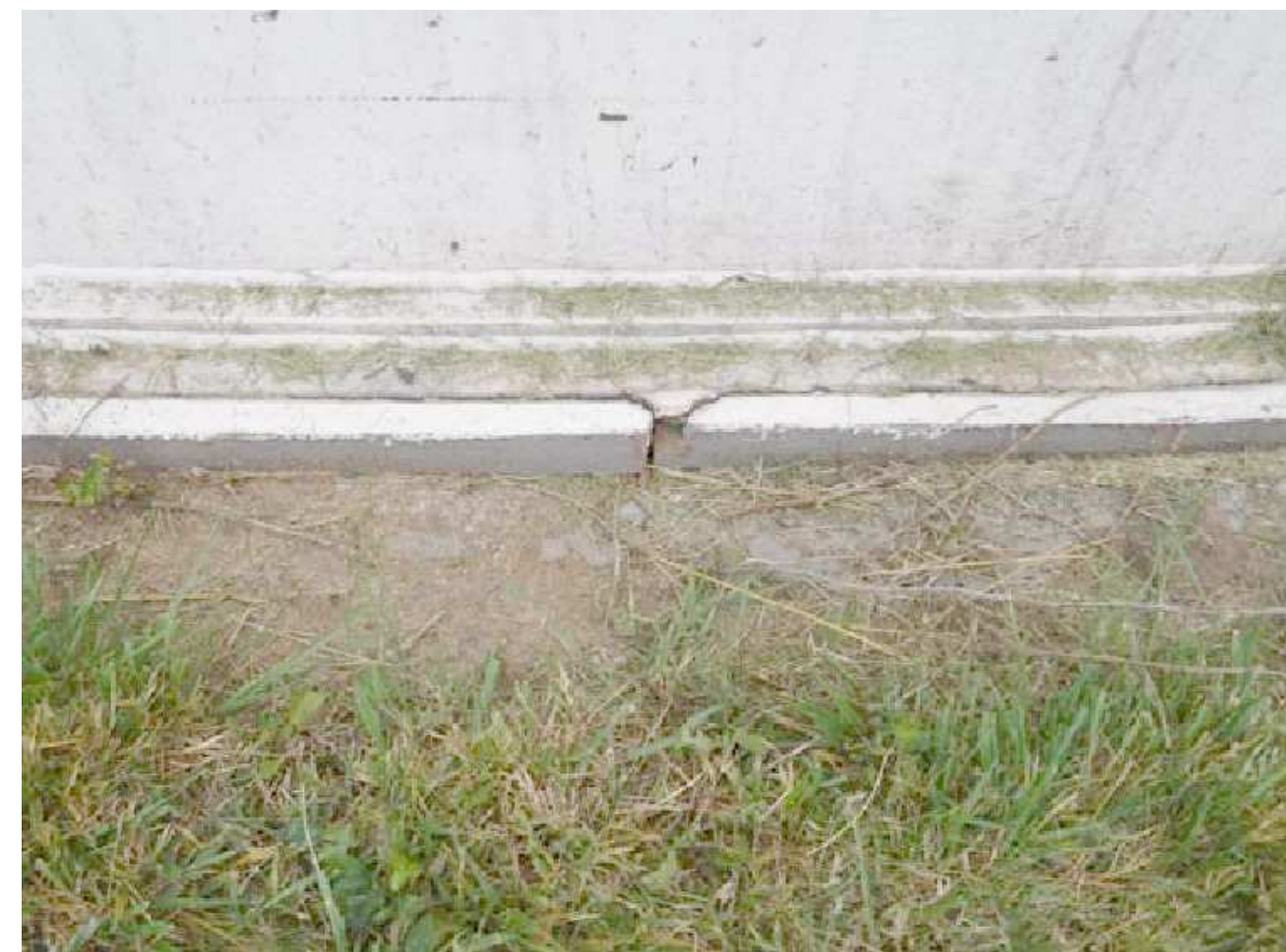
GROUT WITH MINOR CRACKING NO SCALE
