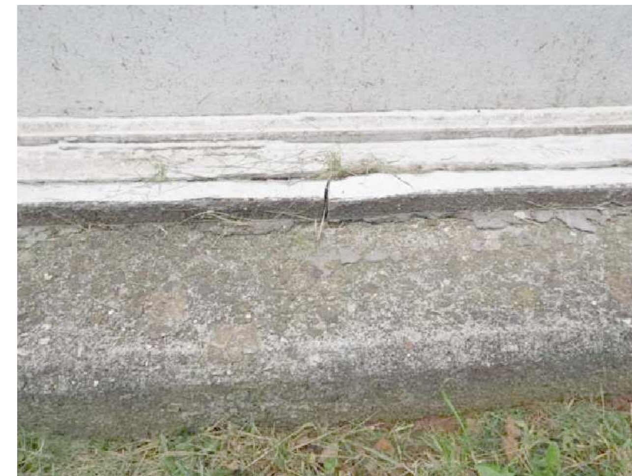
GROUT WITH MINOR CRACKING NO SCALE
