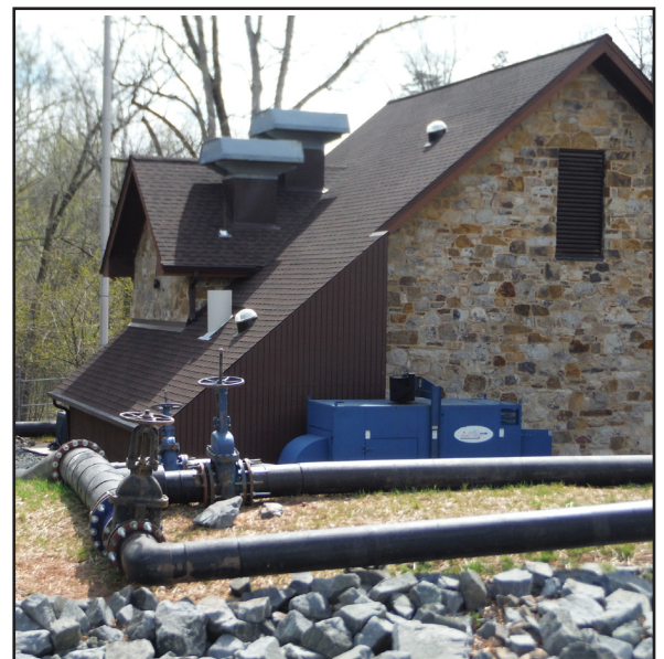
Cattail Branch Pump Station
