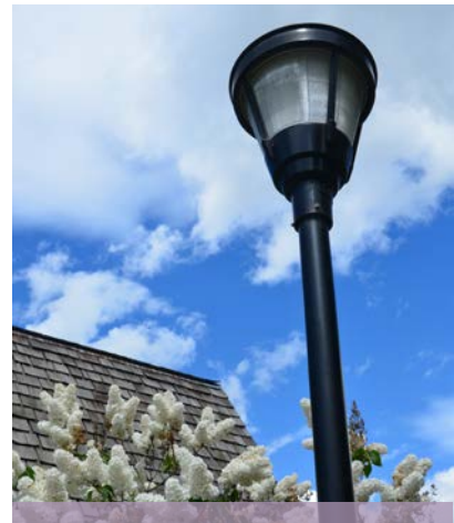
STREET LIGHTS Decorative Street Lights
