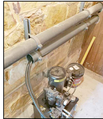
PHOTO 5 - HYDRAULIC LINES NTS
