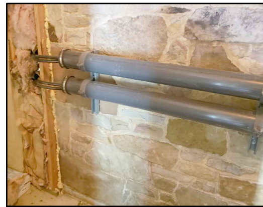
PHOTO 6 - HYDRAULIC LINES NTS
