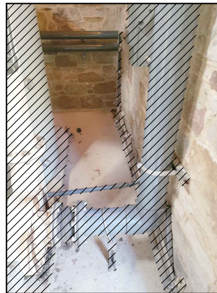
PHOTO 7 - ODOR CONTROL DUCT NTS
