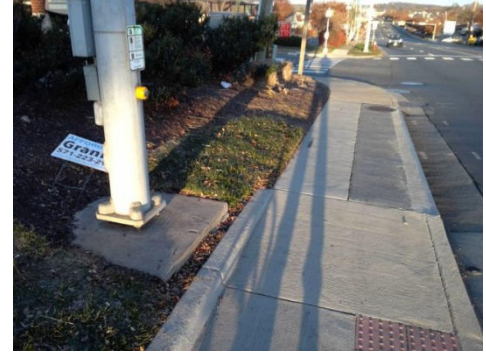
East Market Street & Fort Evans Road: There is not enough clear ground space at the push button and is not at least 10 feet from other pedestrian signals.
