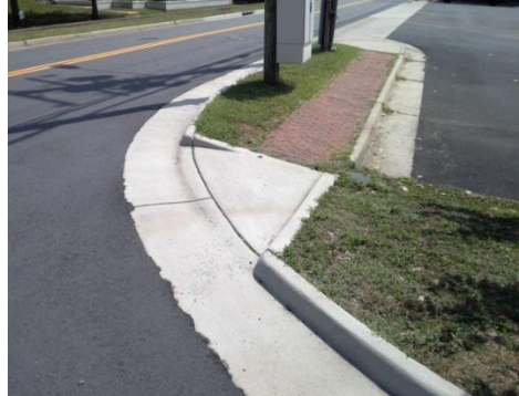
Meherrin Terrace SW: The cross slope is greater than allowed. The slope at the top landing is greater than allowed. The curb ramp does not provide a detectable warning surface which includes truncated domes.
