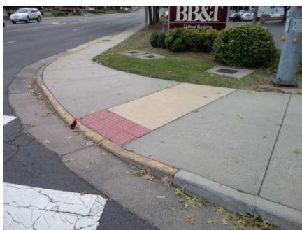
Catoctin Circle & Harrison Street: The transition from the bottom of the curb ramp to the walk, gutter, or street is abrupt.
