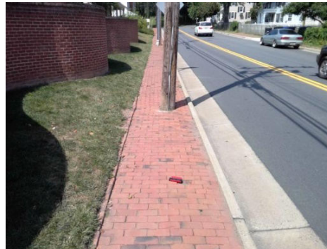
Loudoun Street SW: Sidewalk width at the obstruction is not compliant. Sidewalk cross slope is not compliant.
