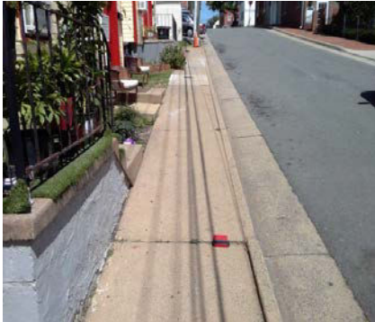
Wirt Street SW: The change in elevation is greater than the recommended value.
