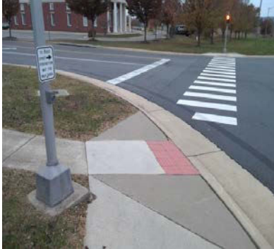
Battlefield & Potomac Drive: Depth of detectable warning not compliant. Push button height, color, and location are not compliant.
