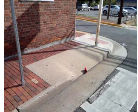
East Market Street: The slope at the top landing is greater than allowed. There are no detectable warnings.
