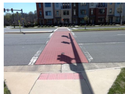
Russell Branch Parkway & Village Market Boulevard: The intersection walking surface change in level height is not compliant. The traffic stop bars are not at the minimum of 4 feet from the crosswalk.
