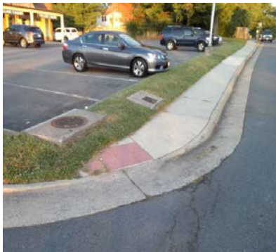
Catocin Circle SW: There is not enough top landing clear length.
