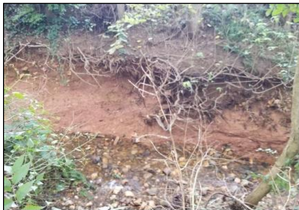
View of undercut bank
