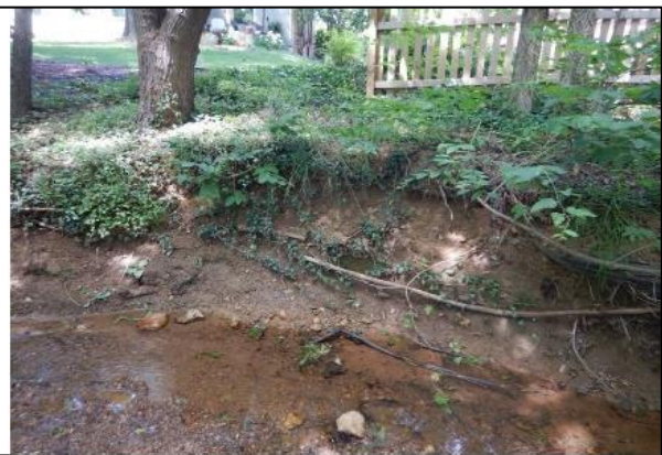
View eroded stream bank, potential property loss
