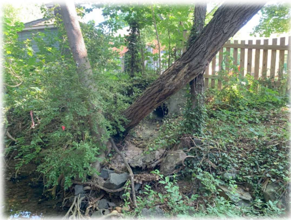
Trees impacting storm discharge
